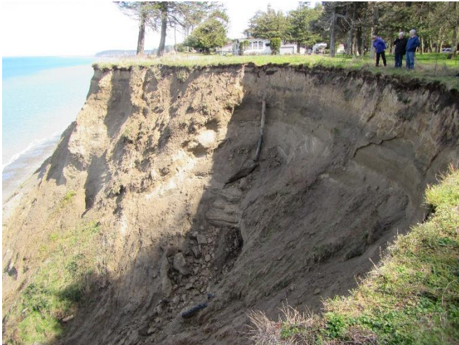
Photo 9. Ravine with broken pipe, looking east.
