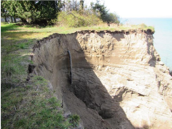
Photo 7. Ravine with broken drainage pipe, looking west.
