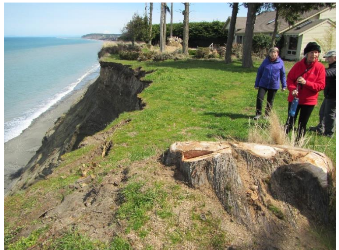
Photo 12. Trees cut at 112 Sea Bluff Lane, and visible cracks along bluff crest.
