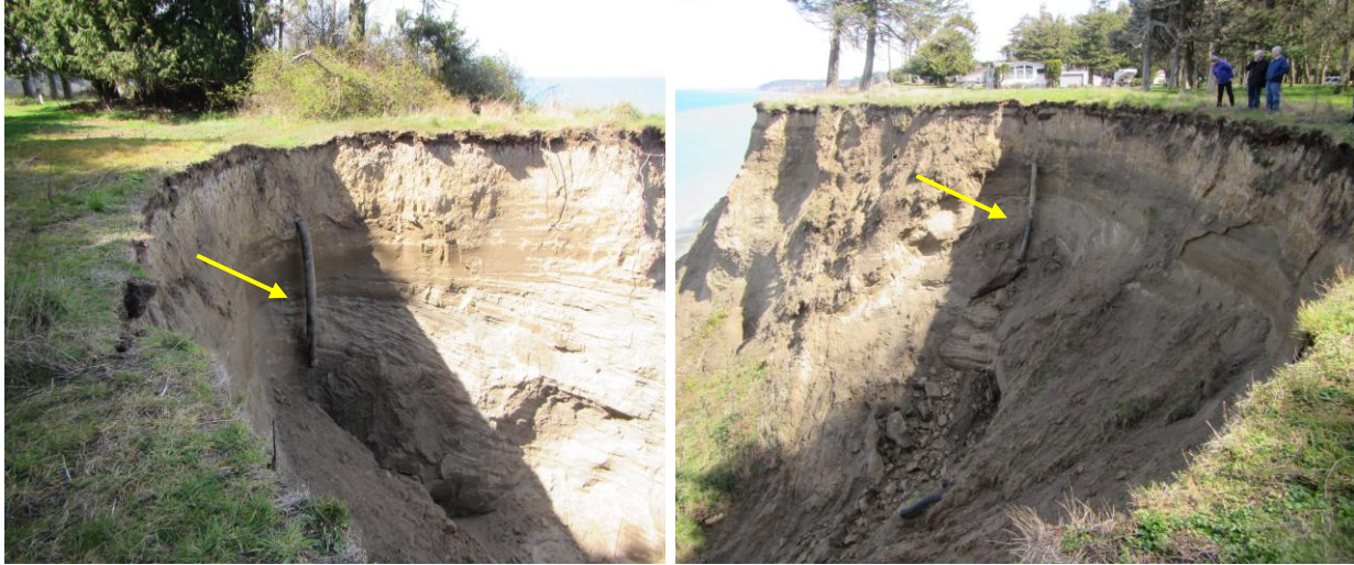
Figure 6. Broken tightlines where overflow drainage expels in ravine northeast of Cypress Circle. Yellow arrow points to tightlines.
