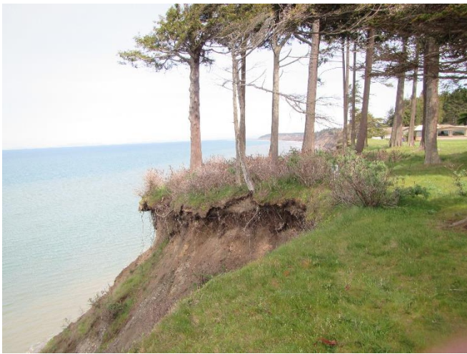
Photo 3. Bluff crest with trees slowing some undercutting.
